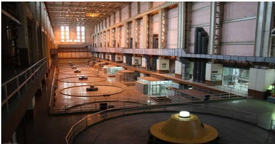
Fig.1.Power house of NSHES
