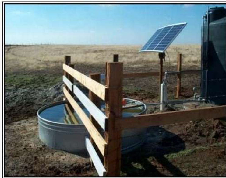
Fig. 4. Solar panel used to discharge water from ground in field.
